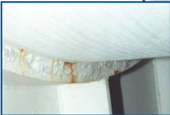
Small rust spots along weld seam on tank bottom – August 2001.
